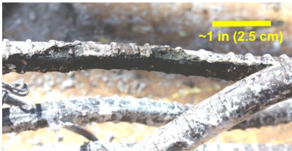
Figure 23. Locally corroded steel in region below mudline. (Bridge C) Note corrosion-related cross-sectional area decrease of bar near top of photo.
