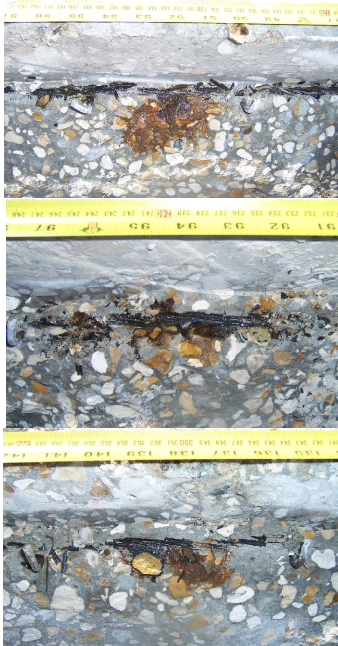
Figure 21. Three different instances of localized corrosion. (Bridge B) Note that the measurement datum for the indicated distances was the waterline.
