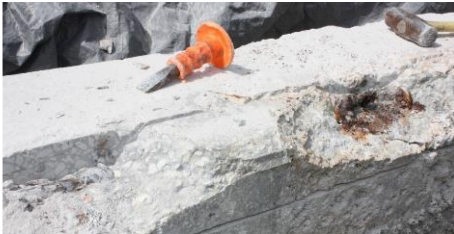
Figure 9. Rust stains in concrete cover observed during bar removal. (Bridge A Pile #2)
