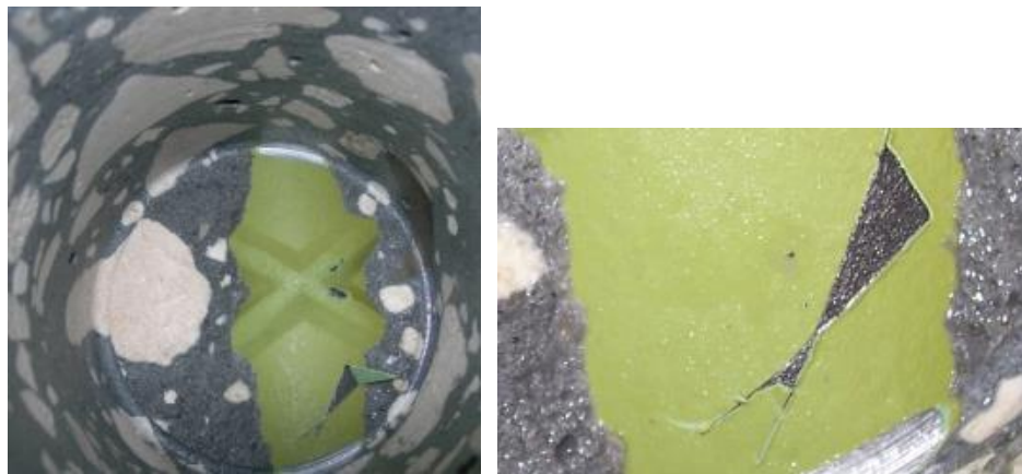
Figure C3. Rebar at core #4 site. Note epoxy cut and easily peeled showing poor adhesion.
