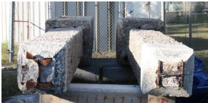
Figure 3. Bridge A piles, end view. Note marine organisms and muck accumulation on each pile's exterior surface everywhere except region below the mudline (foreground).
