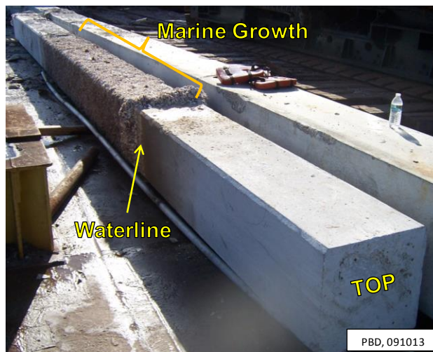
Figure 11. Bridge B pile selected for autopsy. Atmospheric air-exposed end of pile (i.e., top) is in the foreground. Note marine growth between waterline and mudline.
